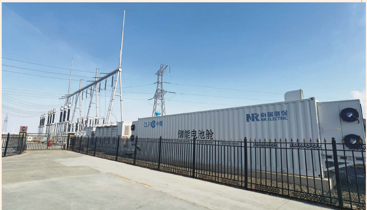
Qian'an III Wind Farm in Mainland China is the first CLP project of its kind equipped with a battery energy storage system.
