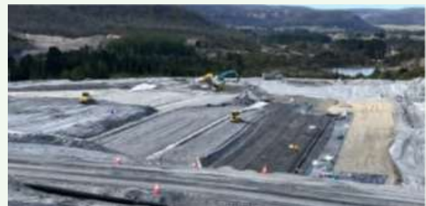
Installation of the Leachate Barrier Management System at the Mount Piper Power Station
