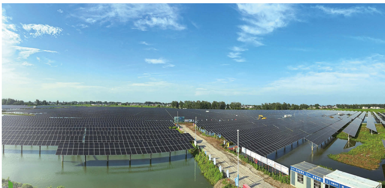
The new Yangzhou Gongdao Solar Power Station in Jiangsu province is equipped with an 8MW commercial use battery energy storage system, the first of its kind in the province.
