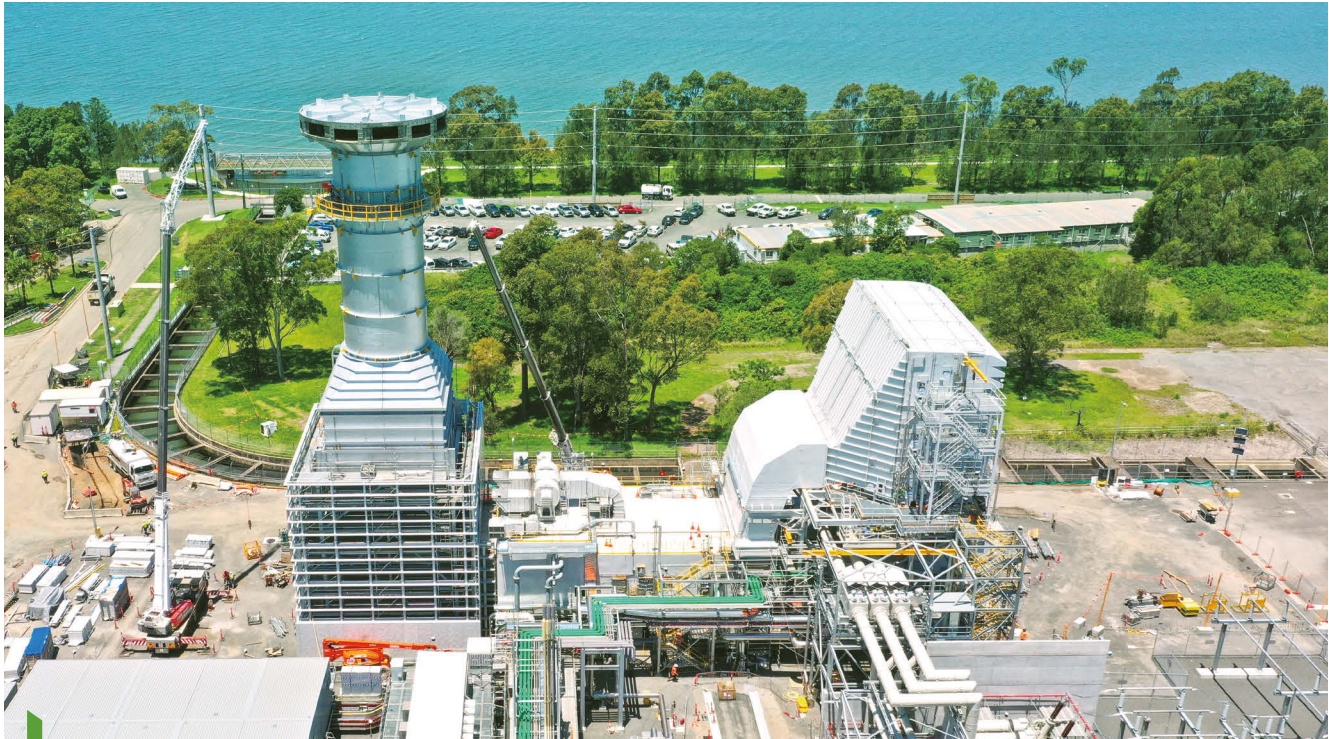
Fast-start gas generation assets like the new 320MW Tallawarra B power station will play an increasingly critical role in providing electricity at peak periods and times of low sunshine and wind in Australia.
